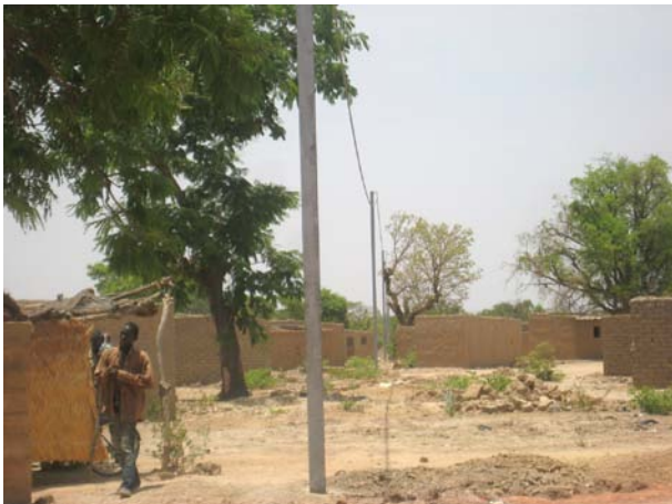
Electric service has come to the ACTS Center
